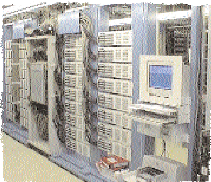
Avaya's Smart Main Distribution Frame features 800 Series twisted pair cable for flawless operation.
